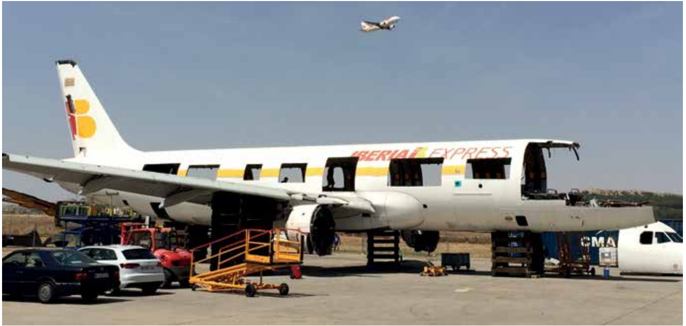
Door sections are carefully removed to make instant cabin door trainers for cabin crew (photo: AELS)
